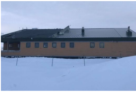
Wales roof damage
