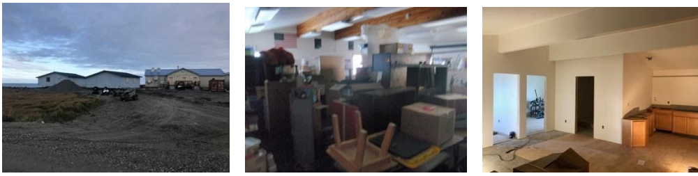
Location of the new SHH housing conversions, before renovations and during renovations
