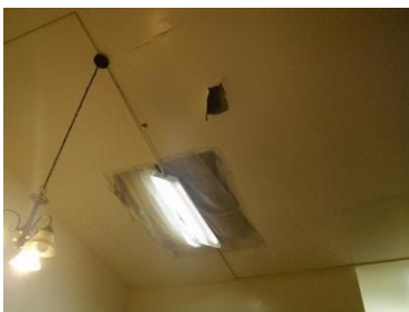
SMK housing water damage
